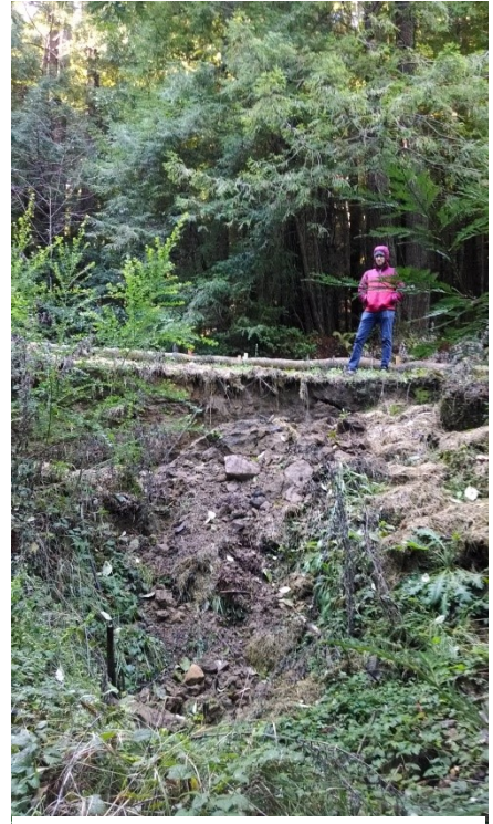
Figure 3. Example of crossing failure: a sinkhole collapsed on the downslope side of Dark Gulch crossing (2015).
