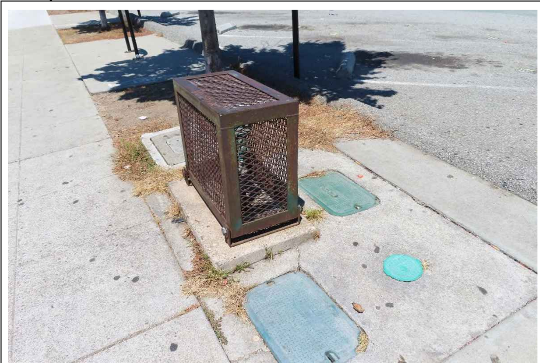
Water Meters and Equipment
