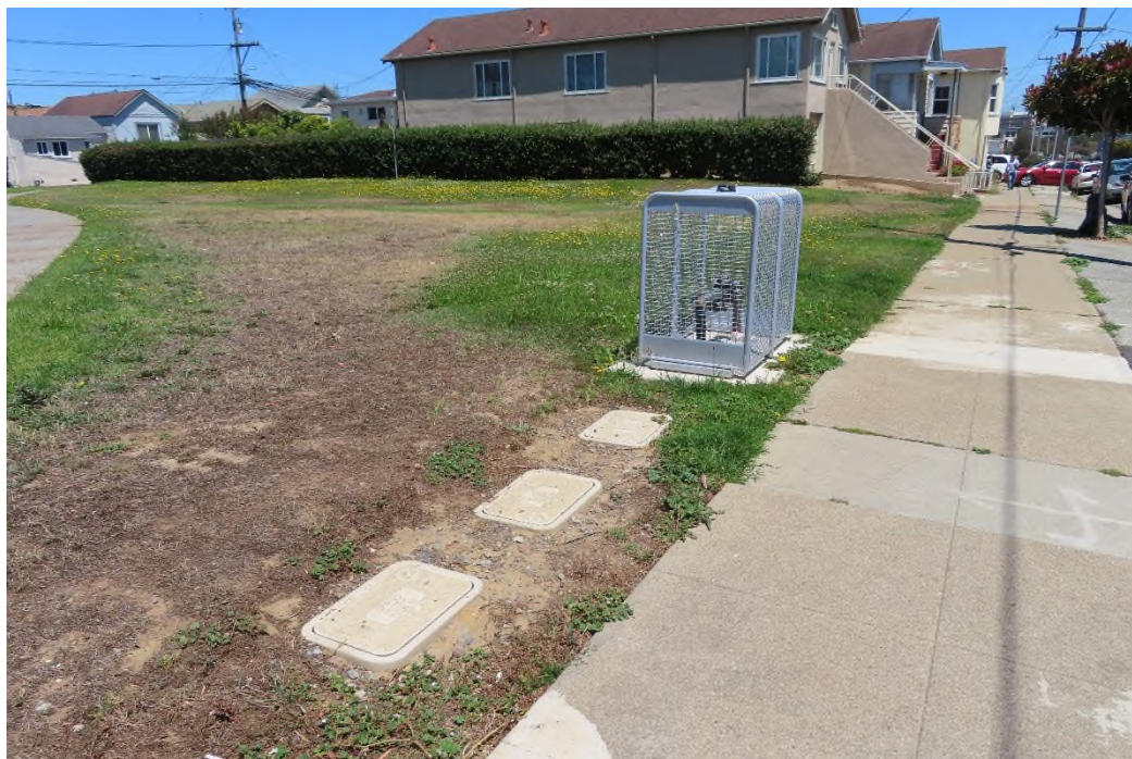
Water Meters and Equipment
