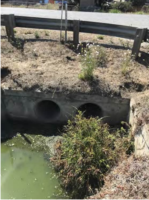
Photograph 13: Double culvert (CWUS-3) for Unnamed Intermittent Creek (OWUS-5) on east side of SR 1.
