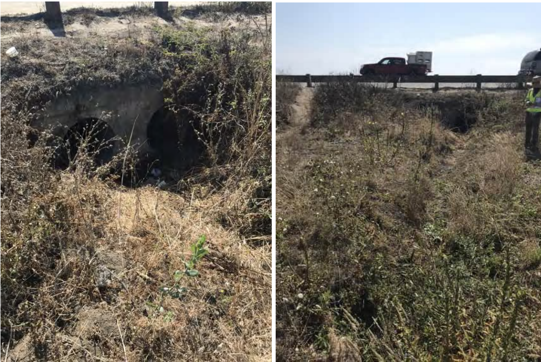
Photographs 28 and 29: Ephemeral creek (OWUS-8) leading to cross culvert (CWUS-6) under SR 1.
